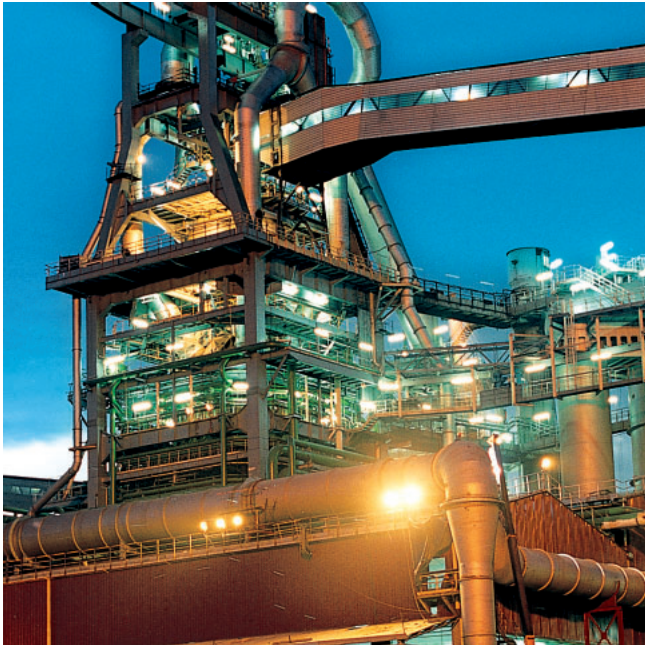
Industrial application: Refinery
